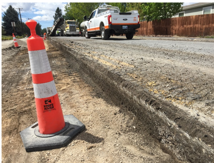
Rebuilding South Canal Blvd. started in March 2018 and is expected to take 13 months.
